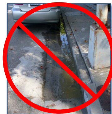
Figure 9: Do not discharge saw cut slurry to the gutter or storm drain system
