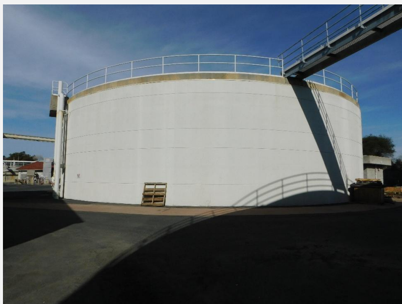
Photograph 9. View of Primary Digester 1, view looking northwest (DSCN_0182).
