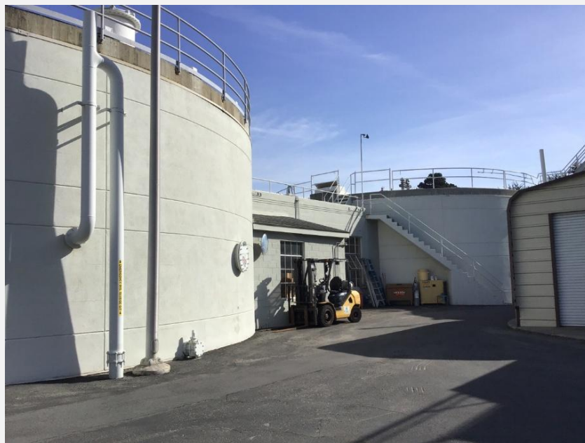
Photograph 2. Digesters 3 (left) and 2 (right), view looking northeast (IMG_11627).
