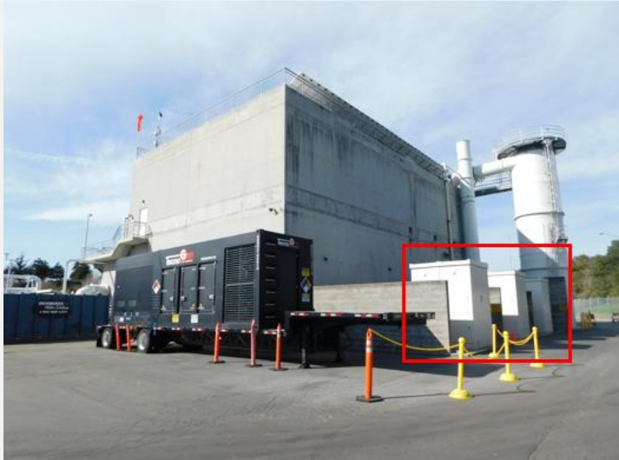
Exhibit 28. View of the Solids Dewatering Building (Map ID 15), showing typical substations less than 45 years of age (Substation 1a/1b) to the east (outlined in red), view looking west (DSCN_0205).
