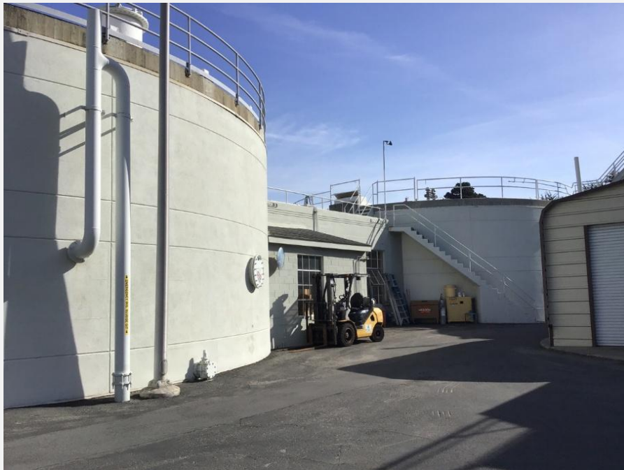
Exhibit 3. Digesters 3 (left) and 2 (right), view looking northeast (IMG_11627).
