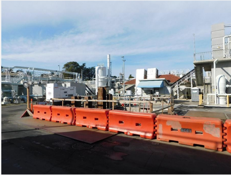
Exhibit 8. Influent Pump Station, view looking west (DSCN_0190).
