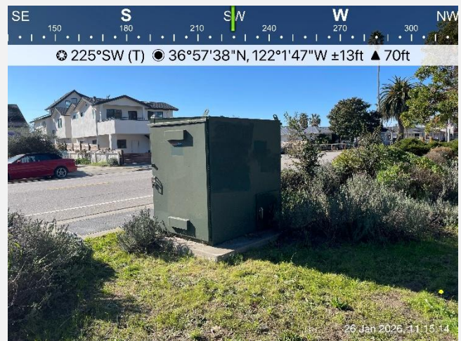
Photo 10. Existing Pacific Gas and Electric 21 kV service box within La Barranca Park and adjacent to Bay Street to be replaced during construction.
