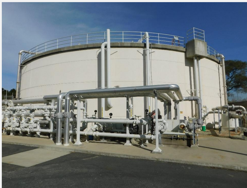
Photograph 11. View of Digester 4, view looking southwest (DSCN_0198).
