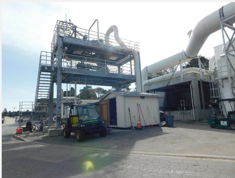
Photograph 23. Partial view of the Odor Control System, view looking southeast (DSCN_0254).
