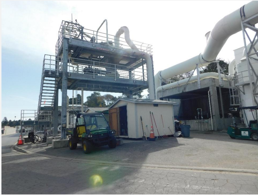
Exhibit 24. Partial view of the Odor Control System, view looking southeast (DSCN_0254).
