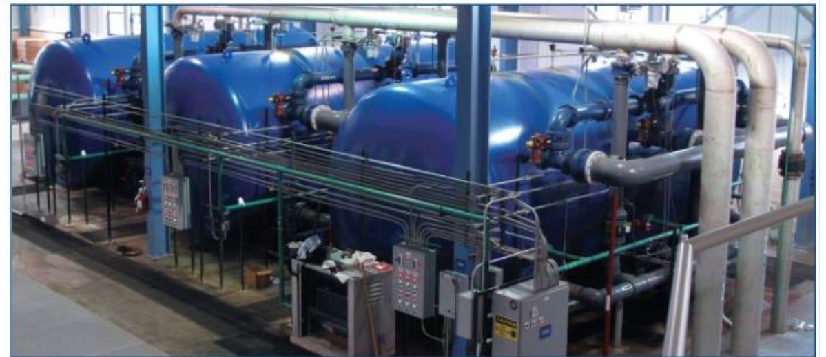
GreensandPlus Pretreatment for RO Filter System 4.2MGD
