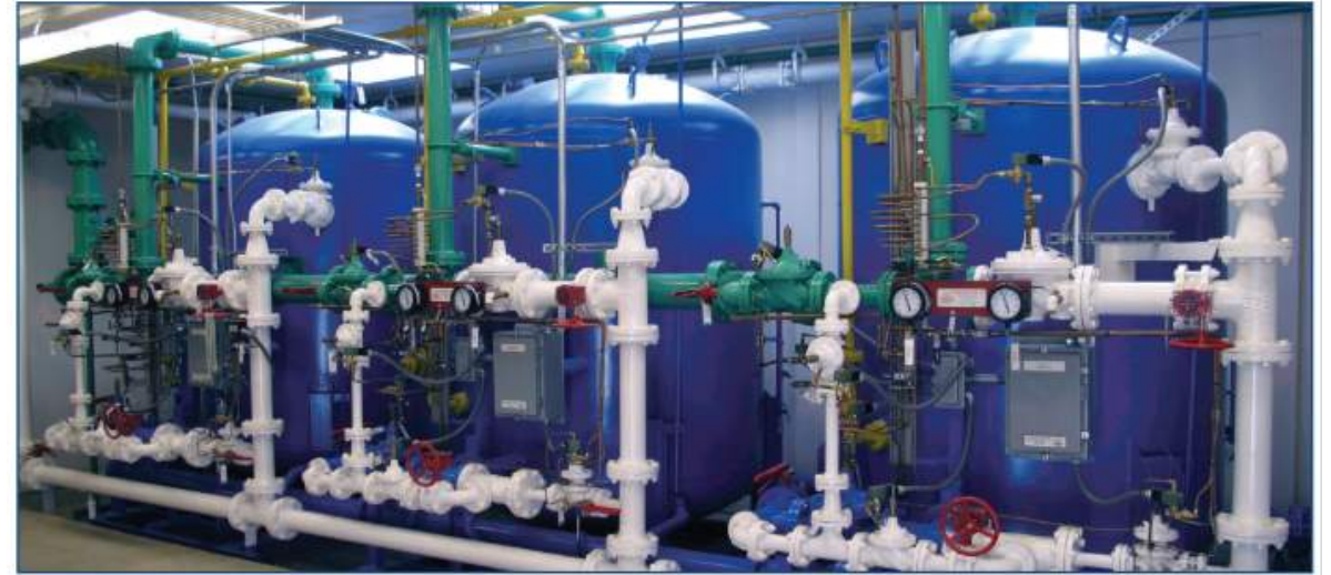
This is an example of the 1.5 MGD municipal filter installation with air/water wash, by Hungerford & Terry.
