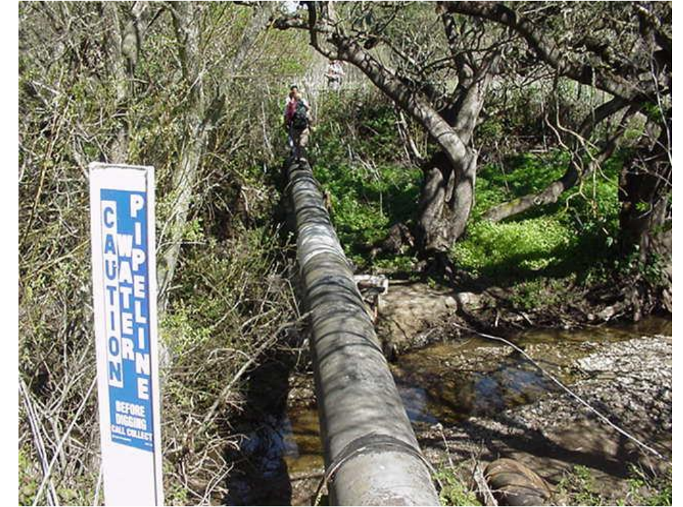
Photo A47 - NCP Reach and NCP Alt. - Pipeline Crosses Peasley Gulch Stream Crossing (NCP-08) Through Central Coast Live Oak Woodland (p.d. 23,900 feet)
