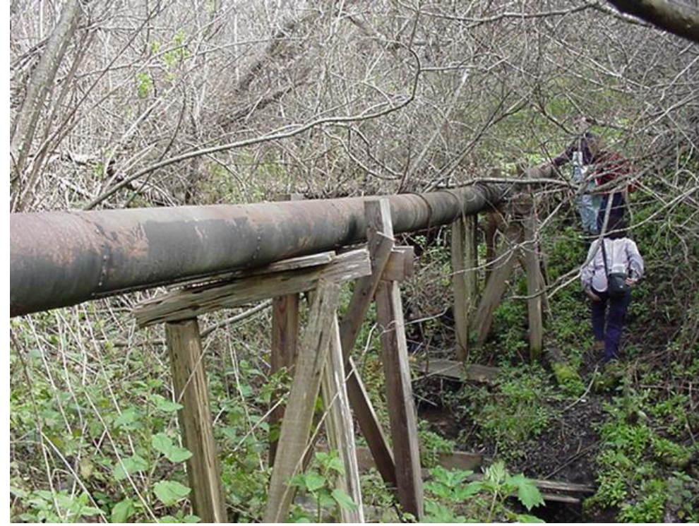
Photo A8 - Liddell Reach and LID-Alt. - Pipeline Suspended Over LID-03 Stream Crossing (p.d. 7,500 feet)
