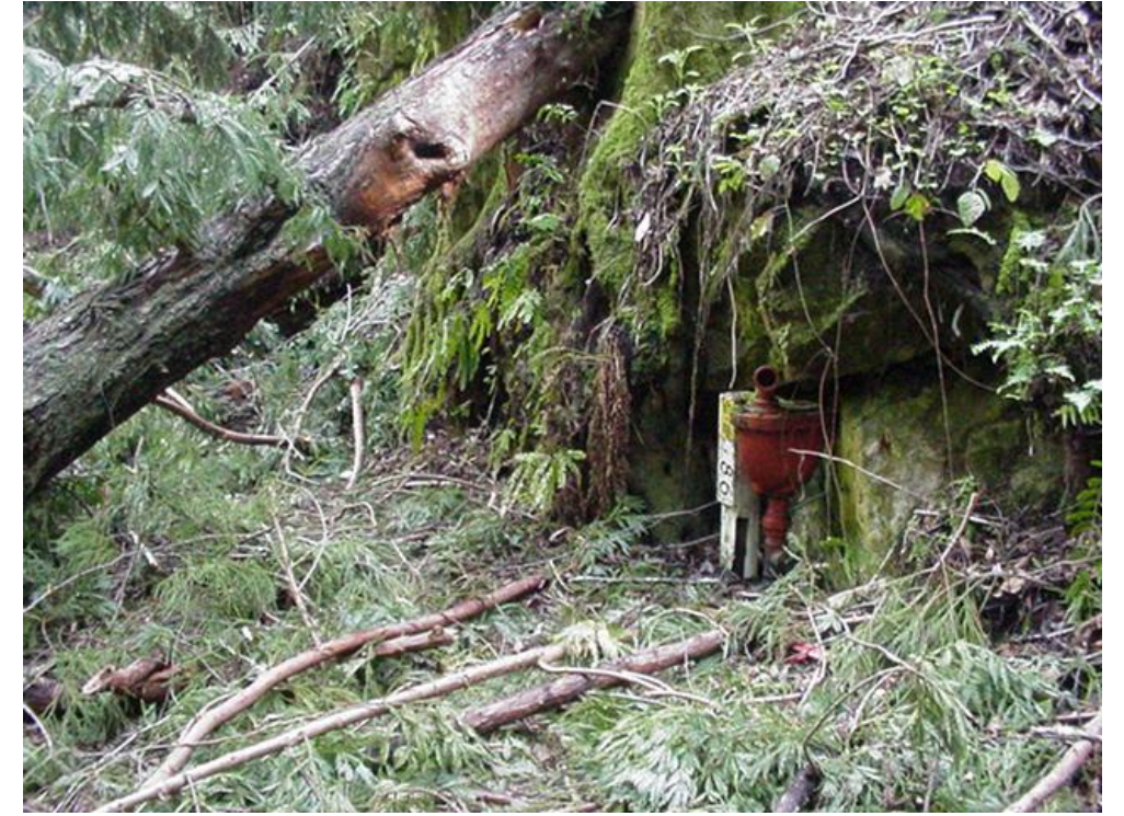
Photo A15 - Laguna Reach - Blow Off Valve to the Left of the Road
