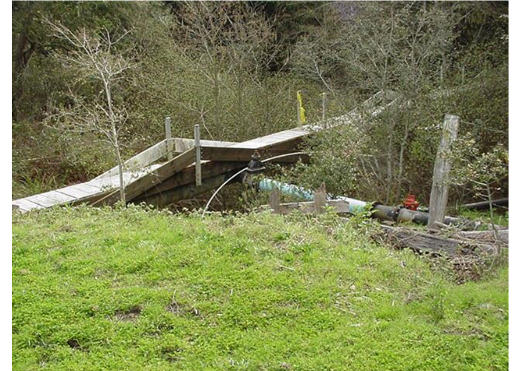
Photo A21 - Laguna Reach - Intersection of Laguna and Liddell Pipelines at LAG-04 Crossing on "Y" Creek
