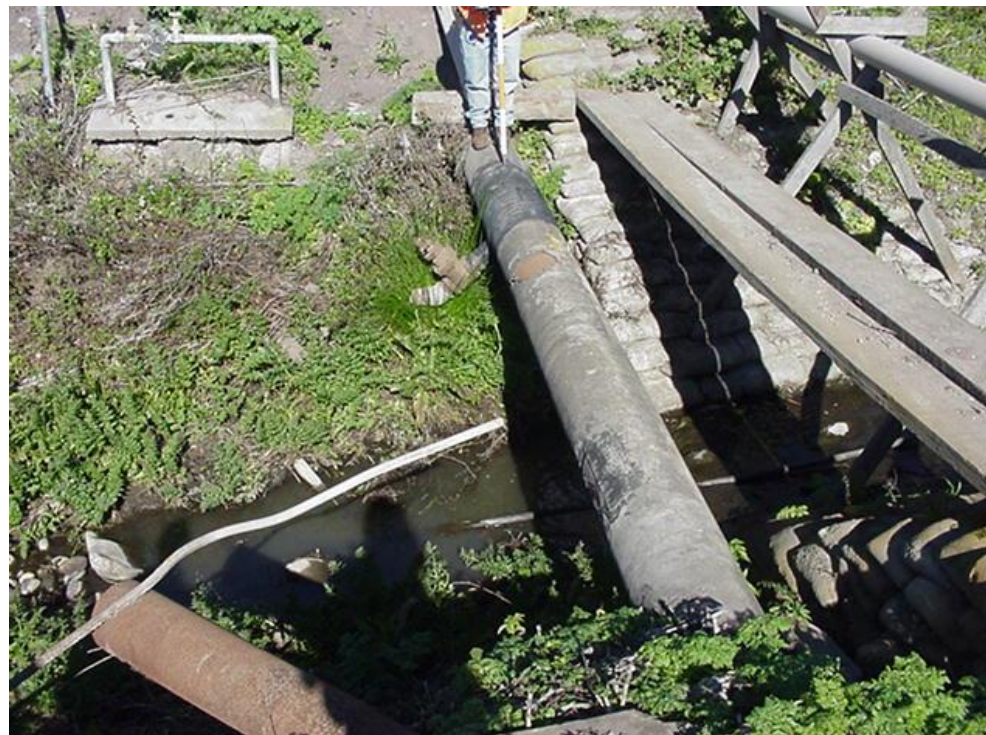
Photo A43 - NCP Reach and NCP Alt. - Pipeline Crosses Gordola Creek(NCP-03) Stream Crossing (p.d. 8,000 feet)
