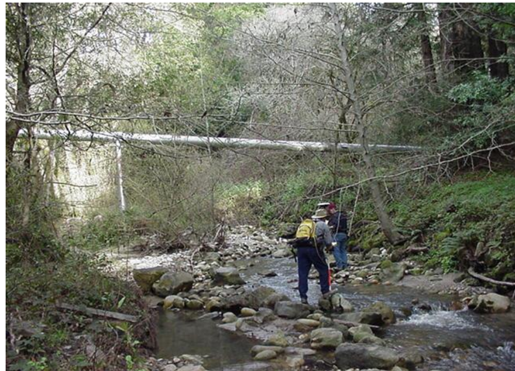
Photo A25 - Laguna/Liddell Reach - Pipeline Suspended Over LAG/LID-02 Stream Crossing (p.d. 2,600 feet)
