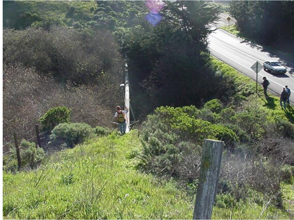
Photo A40 - NCP Reach and NCP Alt. - Pipeline Suspended Over Majors Creek (NCP-02) (p.d. 4,800 feet)
