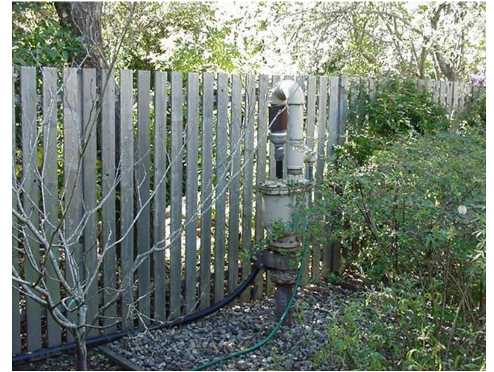
Photo A53 - NCP Reach - Air relief valve in residential yard (p.d. 38,000 to 40,000 feet)
