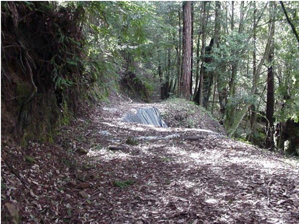
Photo A16 - Laguna Reach - Wash Out Area from 1998. Pipeline Exposed Beneath Plastic Sheetting Between Street Crossings LAG-02 and LAG-03
