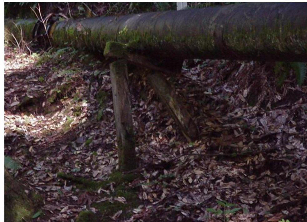
Photo A35 - Majors Reach - View of Collapsing Trestle Supporting Pipeline (p.d. 500 to 2,000 feet)
