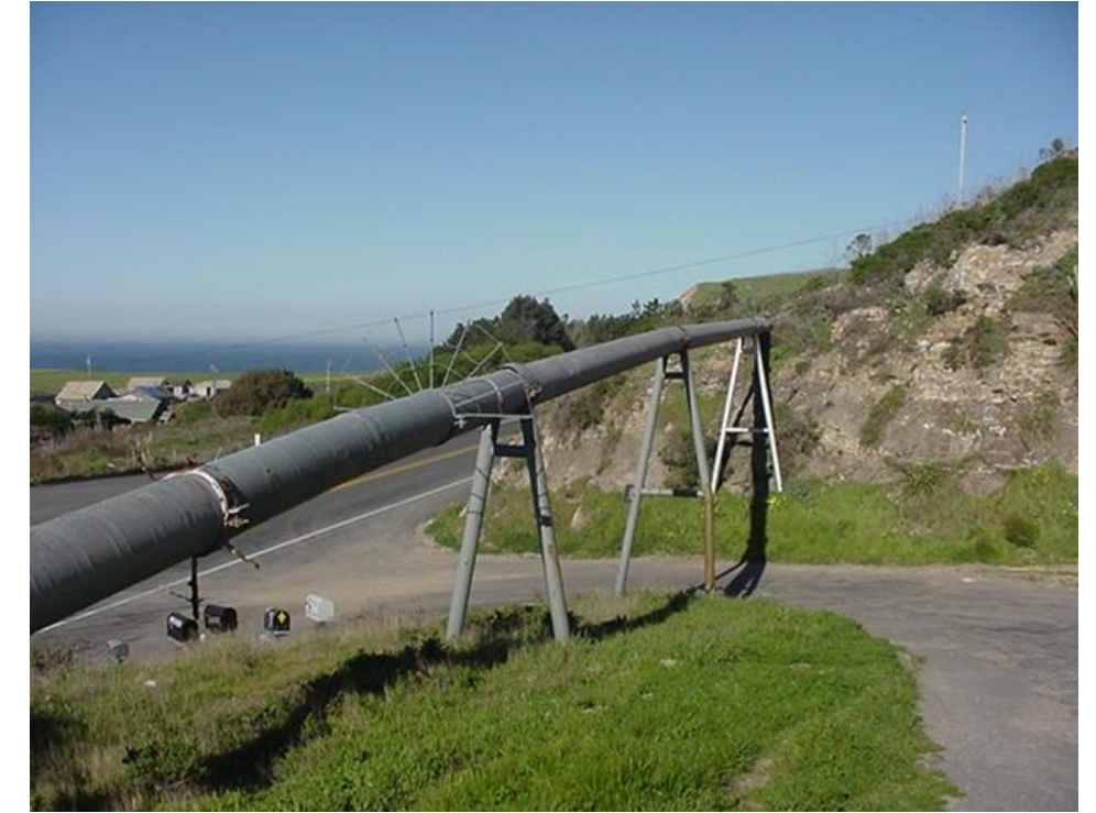
Photo A41 - NCP Reach and NCP Alt. - Pipeline Suspended Above Ground at Back Ranch Road and Hwy 1 (p.d. 3,600 feet)
