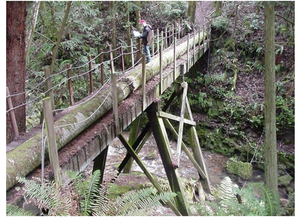
Photo A18 - Laguna Reach - Suspended Pipeline Over LAG-03 Stream Crossing (p.d. 6,600 feet)
