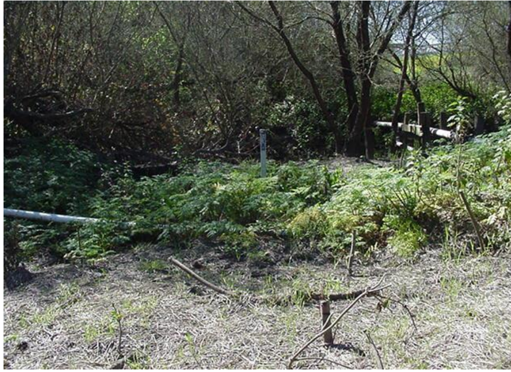
Photo A45 - NCP Reach and NCP Alt. - Pipeline Crosses Sandy Flat Gulch Stream Crossing; Previous Pipeline Breach Location (NCP-07) (p.d. 21,200 feet)
