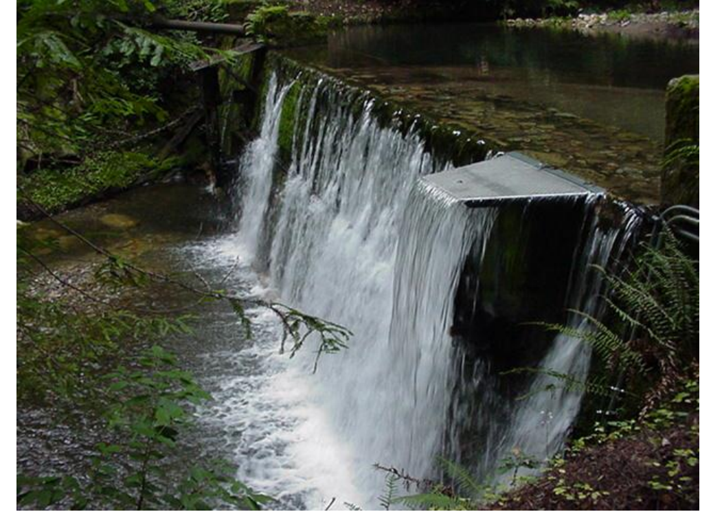
Photo A12 - Laguna Creek Diversion Dam – Note Two Covers for Flow Release Valves
