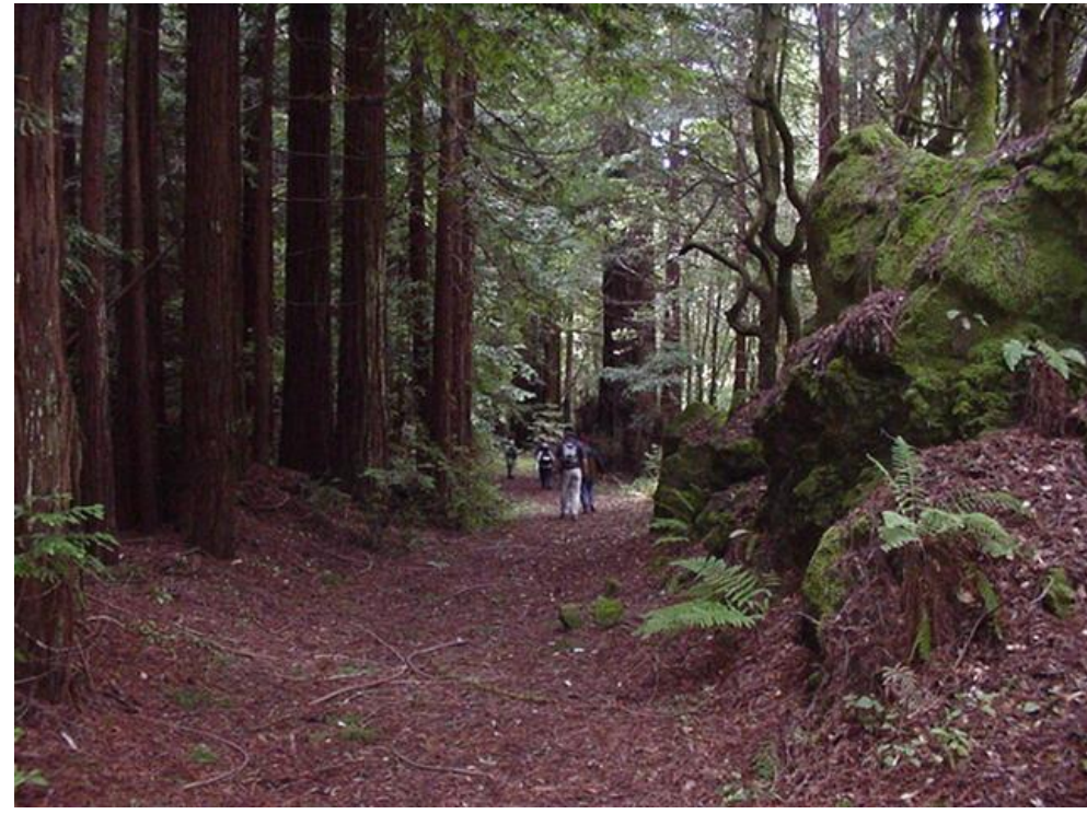
Photo A17 - Laguna Reach - Typical Second Growth Redwood. Pipeline Buried in Roadway. (p.d. 5,000 to 6,000)
