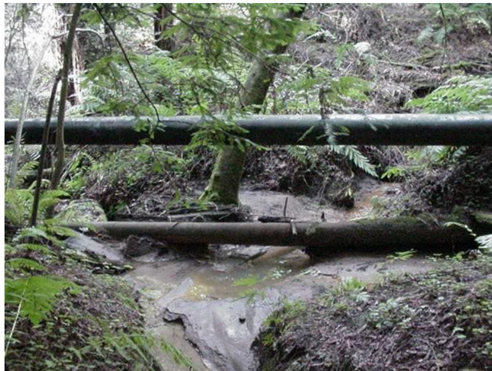
Photo A4 - Liddell Reach - Pipeline Crosses Discharge from Quarry Sedimentation Ponds (p.d. 1,500 feet)
