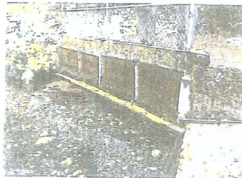
Photo 3.2 - Laguna Creek Intake Screens
